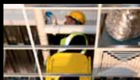
Confined Space Guardrail
